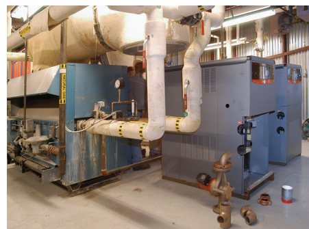
The first two new boilers, at right, were installed as one of the existing boilers continued to operate. Minimizing downtime was critical.
