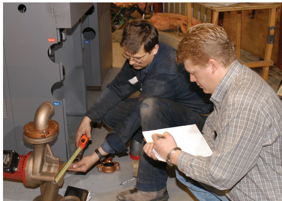
Plumber Jarek Padjesek, left, and project manager James Hill take measurements to determine pump location.
