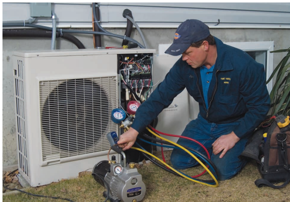
Installation manager Kurt Lehmann checks the operation of the condensing unit. (David Szabo photo)
