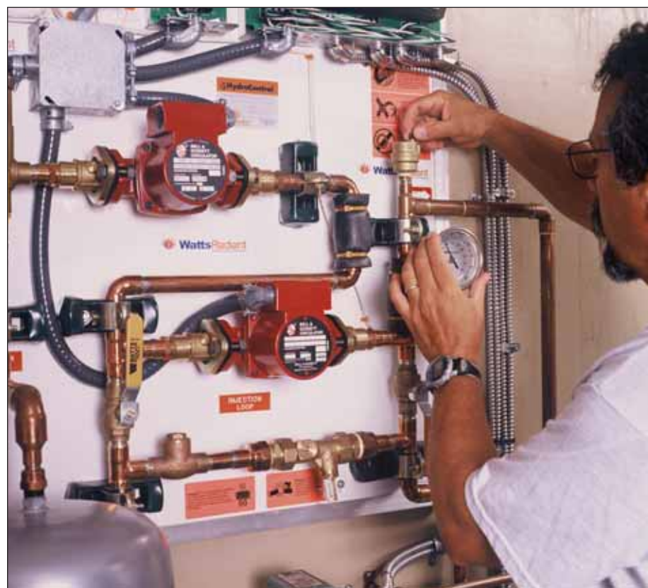
Here, Yates checks a wall-mounted, direct-vent, propane-fired Mini-Therm boiler by Laars Heating Systems, and a pre-manufactured "HydroControl" injection panel made by Watts Radiant.
