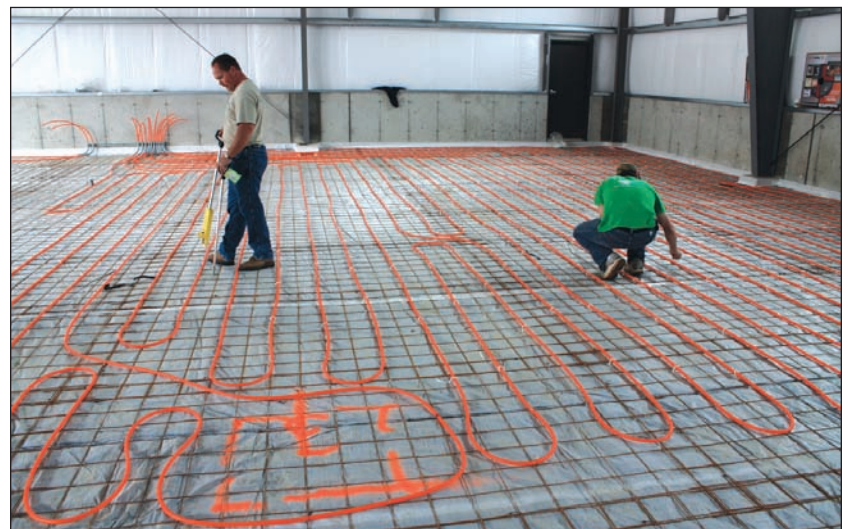
Ciardelli recently branched into radiant heating and snowmelting, and to gain more experience with the technology, installed radiant floor heating in its new facility.
