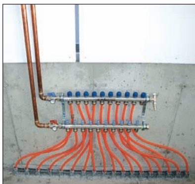
A Watts Radiant manifold distributes heated water to the loops of PEX in Ciardelli's new facility.
