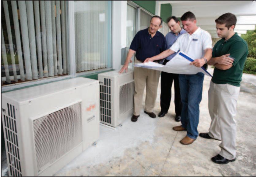
Looking at completed installations at the Marion Center are (from left to right) Tropic Supply's Charley Del Vecchio (CEO), Chuck Del Vecchio (president); Bob Garrison, president of Garrison Mechanical, and Alex Rodriguez, marketing manager of Tropic Supply.
