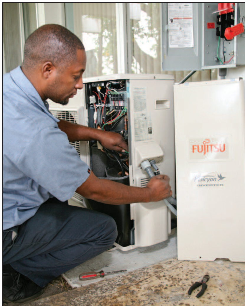
Garfield Thompson, Garrison Mech. technician, completes electrical connections to a condensing unit.
