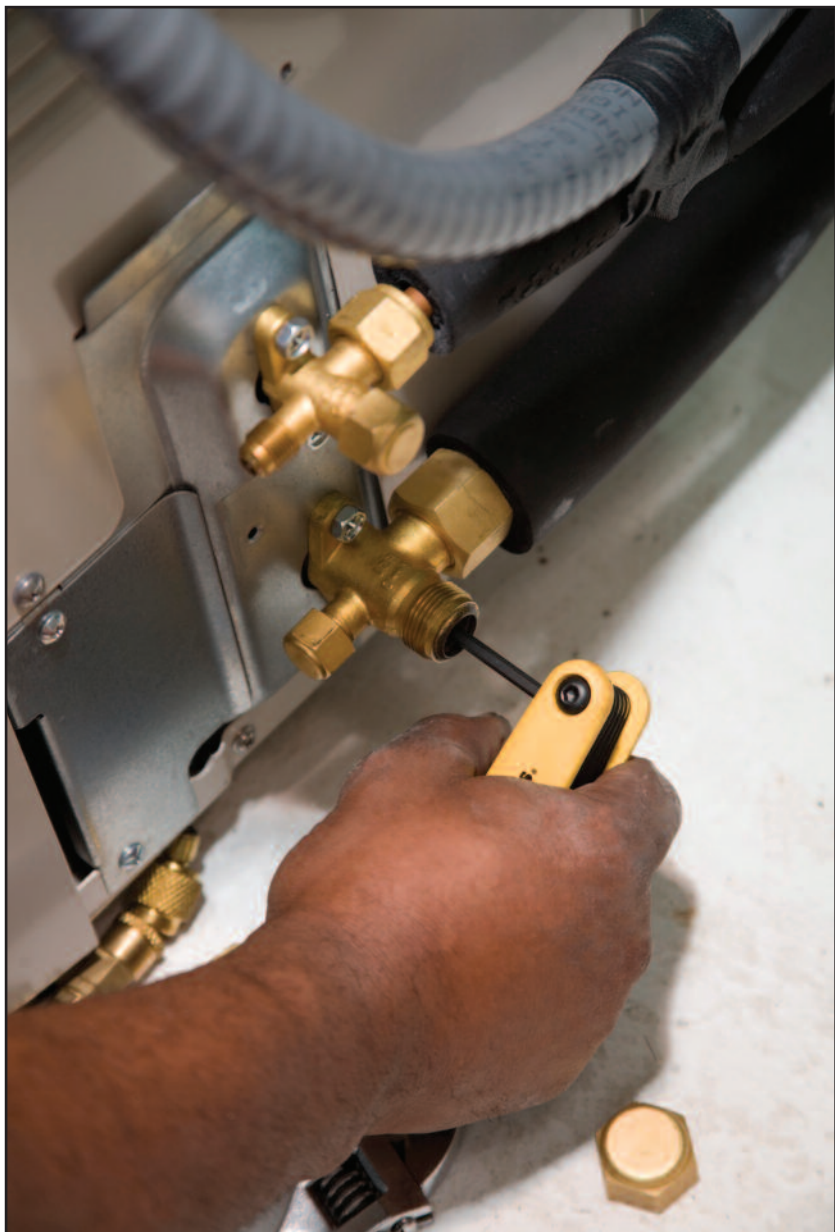
A technician opens the service valve to charge the system.
