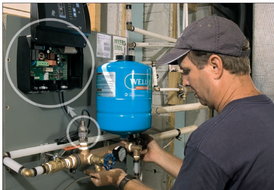
The pressure transducer maintains constant pressure by giving the controller a pressure signal that's used to increase or decrease the speed of the pump to sustain a constant, preset pressure in the 3,000 to 10,700 rpm range for gradual build-up or slowing-down of the motor for continuous maintenance of a desired pressure.
