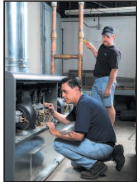
Dave Carlson (right) and a DCM Service technician inspect the Laars Pennant boiler during a pre-fire system check at Los Alamitos.
