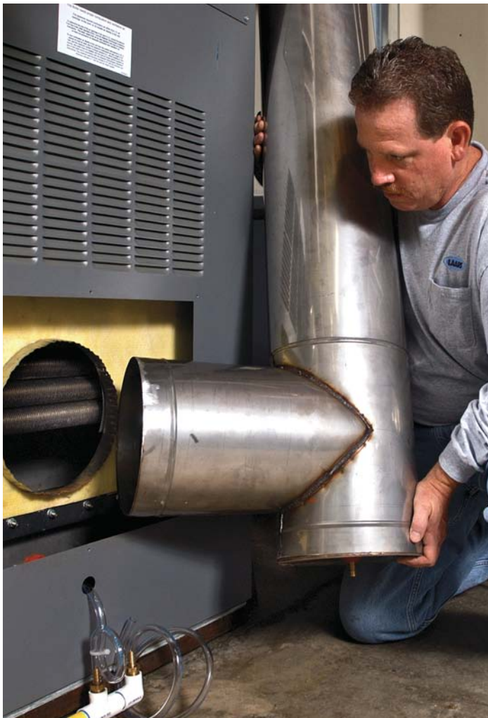
Dave Carlson installs a stainless steel vent for the Los Alamitos facility’s Rheos+ boiler.
