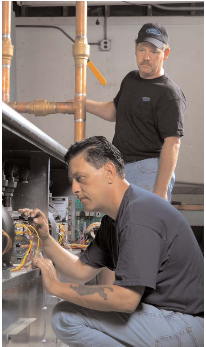
Dave Carlson (right) and a DCM service technician inspect the Laars Pennant boilers during a pre-fire system check at Los Alamitos.
