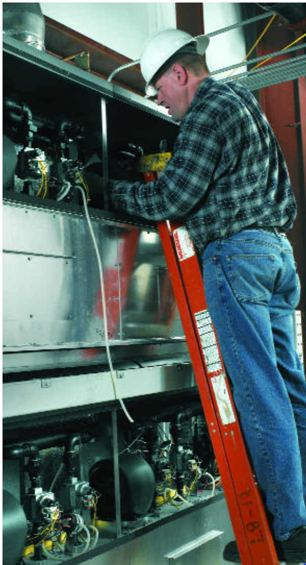
All arteries of the extensive heating system lead to and from the strategically-located mechanical rooms, where, at the heart of the system, are two stacked 1.5 million Btu, fan-assisted, sealed combustion boilers.
