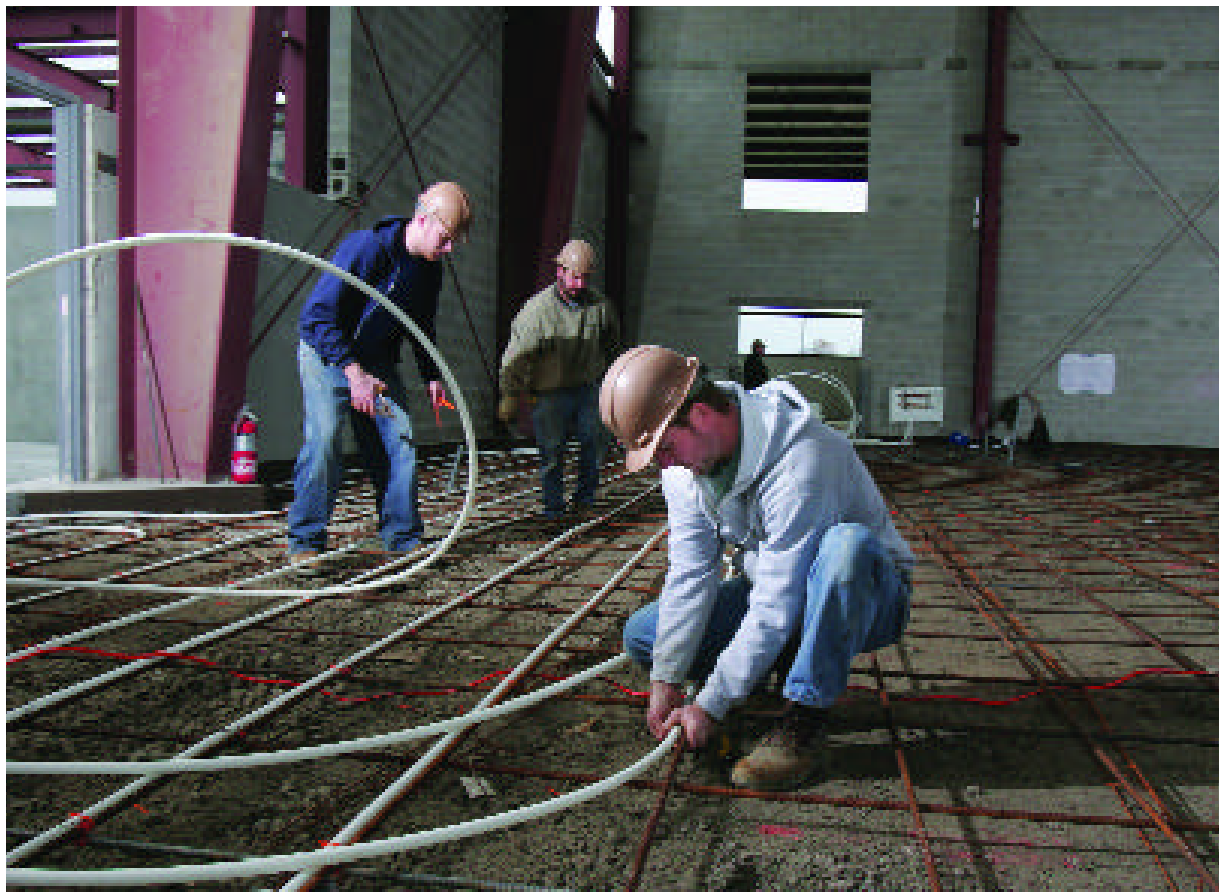
For this one-zone, seven-manifold system, the radiant design team used 55,000 lineal feet of 3/4-inch PEX tubing.
