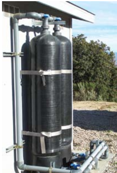
Hahn Family Wines chose a template-assisted-crystallization system to improve process-water quality.
