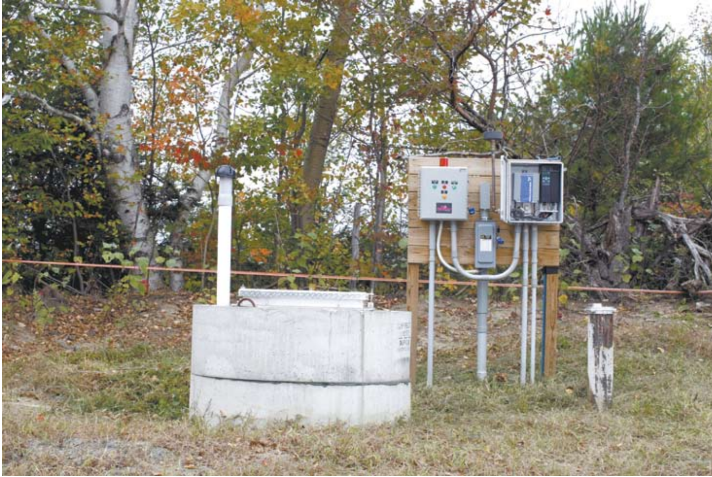
No building required – a complete set of controls and an alarm for a deep well submersible and submersible booster pump with complete climate control for a seven-home subdivision.
