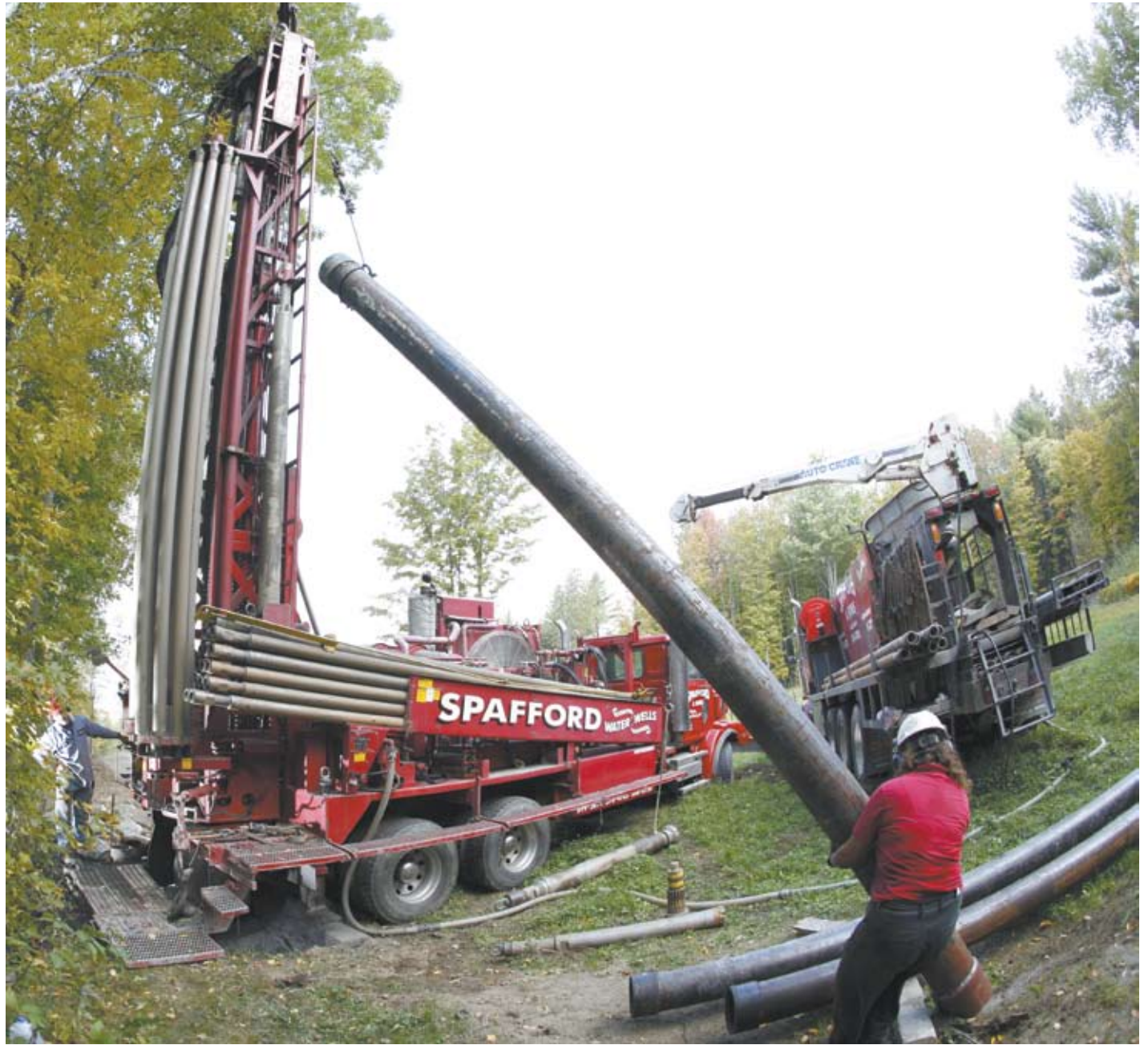
Mellisa “Diesel” Mullen handles a piece of 8-inch with a drive shoe to start setting the 60-foot casing required to get to competent rock.
