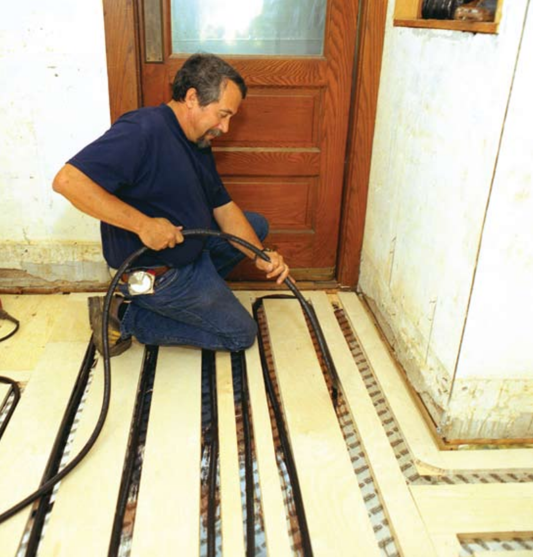
Dave Yates installs Onix tubing in SubRay channels.
