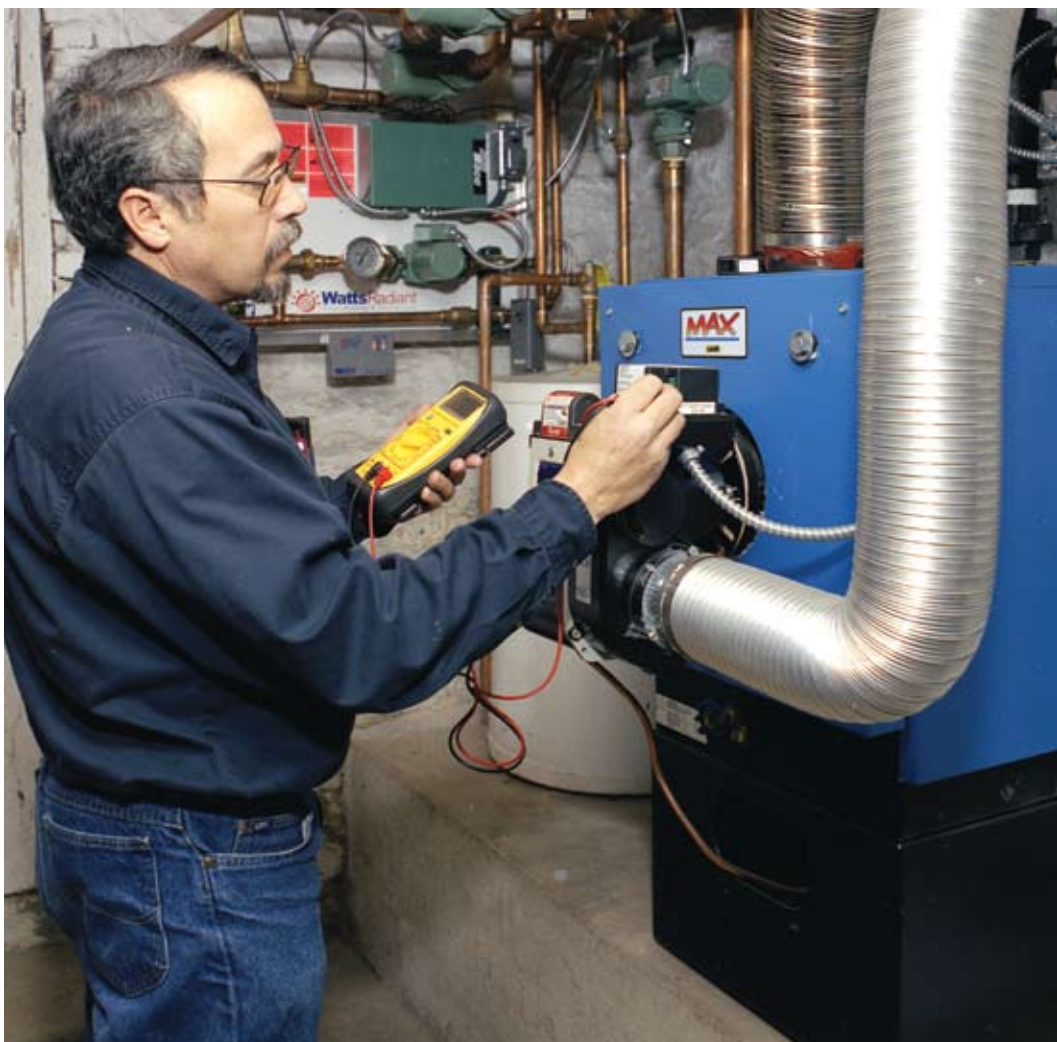
Dave Yates of F.W. Behler Inc. checks on the operation of the oil-fired boiler that was installed as part of the only major renovation of one Pennsylvania home.
