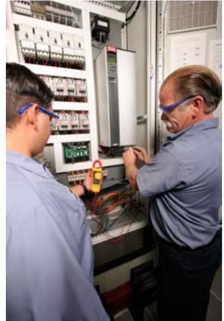
PumpMan, Inc., field service supervisor Mike Woodward, left, and lead mechanic Elmer Brady test the control panel.
