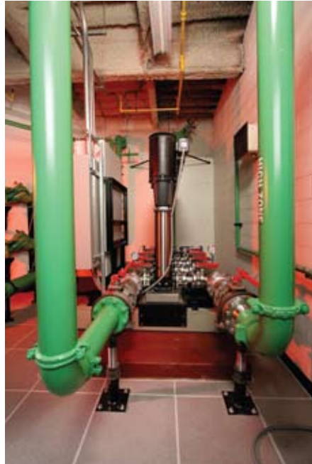
Figueroa at Wilshire's new booster pump system, variable speed booster pump system and low zone pressure regulator system installation completed.
