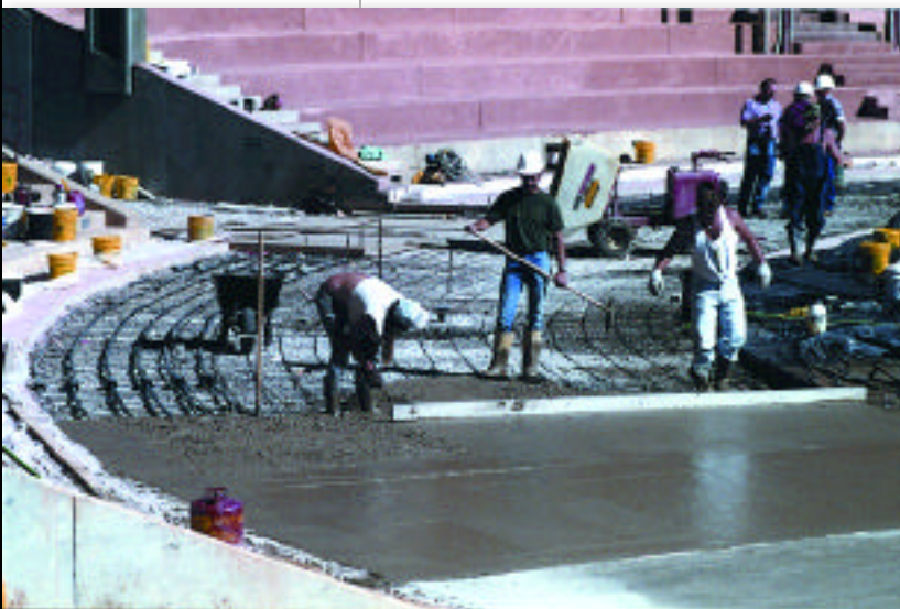
PHOTOA. Installation of 29 miles of radiant tubing underneath the field at Gillette Stadium in Boston.
