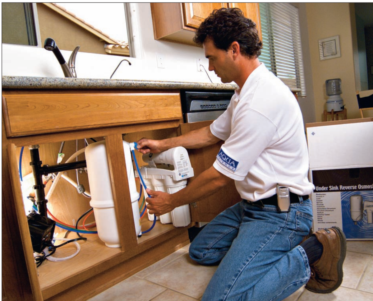
Derek Sajdak, president of Aqua Science in Phoenix, Arizona, completes a storage tank connection for a manifold reverse osmosis unit.
