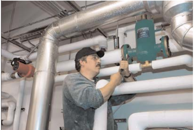
A technician adjusts a Caleffi air separator in a commercial installation that Eayrs did for a local ice rink on the Spit in Homer, Alaska.
