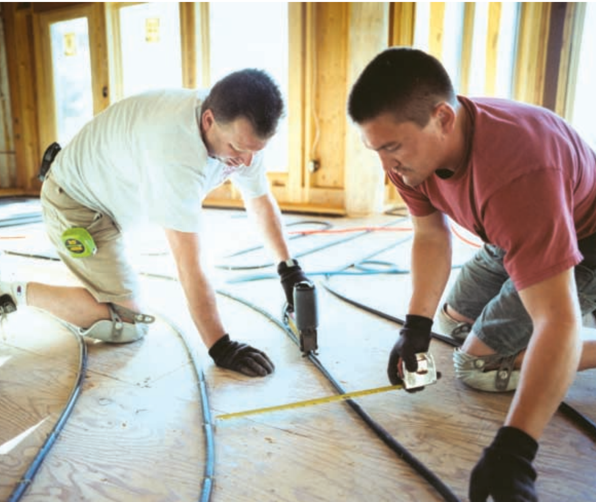
Davis Plumbing and Heating employees install Onix tubing in the interior of the Chambers home. The contractor takes a systems approach and works with the same components on most of its jobs.
