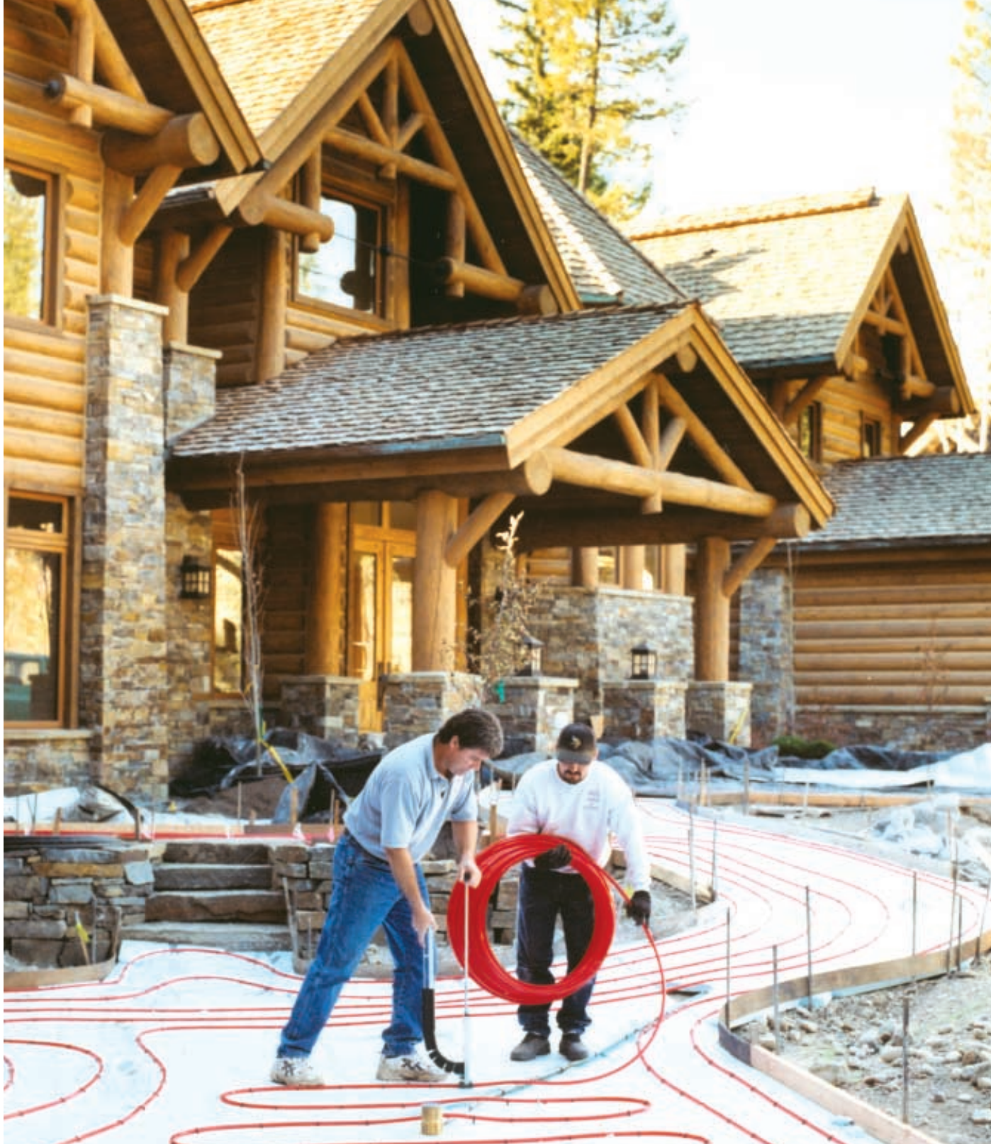
Doug Davis and one of his employees install PEX tubing for a snow-melt system at the Bernstein residence in Montana.
