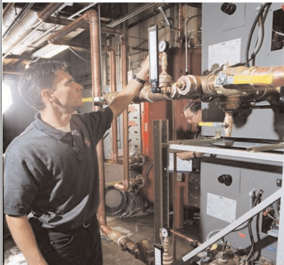
Improved efficiency and reduced emissions are not the only measures of "high-performance" in boiler systems. Maintenance convenience and accessibility are also important considerations.
