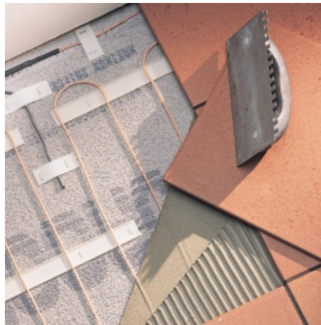
Thinset is applied over the wire mesh of an electric radiant heat system, then the tiles are placed (left). The same basic techniques are used with concrete, hydronic tubing, and laminate, wood or sheet flooring (below).
