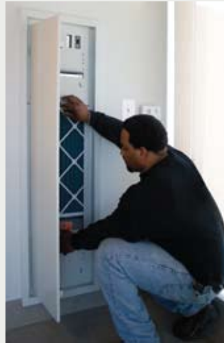
A technician completes the installation of a vertical-stack unit in an upscale condominium.
