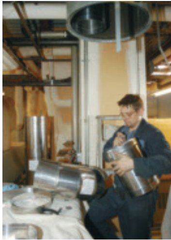
Jarek Padjasek makes preparations to run new stainless steel venting into the existing venting plenum for support.
