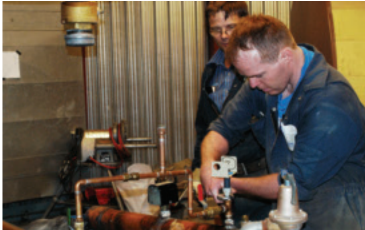
Jarek Padjasek and Kyle Kellar (front), plumbing technicians, T&P, tear down the old boilers in the demolition phase.
