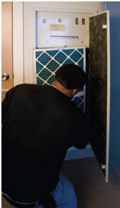
A technician completes the installation of a ClimateMaster TRM vertical stack unit at The Alta at Thomas Circle.
