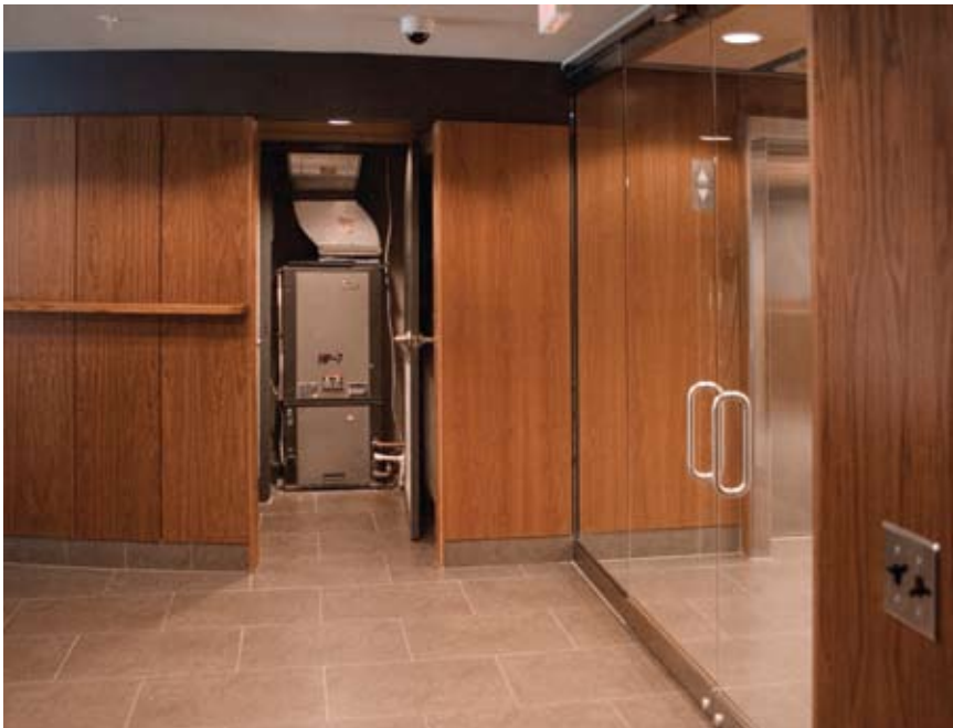
A Tranquility 20 vertical packaged unit in a small closet in The Alta at Thomas Circle's second-floor lobby.
