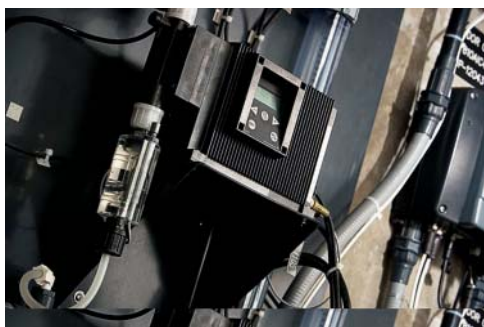
A digital dosing pump used for hypochlorite delivery in the Durham facility.
