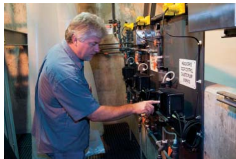
The output of this alum pump can be sized to match current and future plant demand by simply pushing a button.
