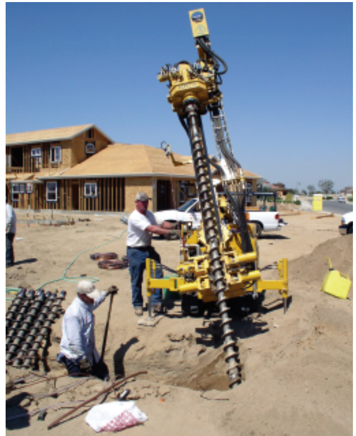
Bore-holes are drilled into the side of a manifold pit, connected by trenching.
