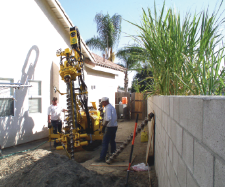
The proximity to the house and lack of spaciousness during this California installation made the diagonal boring method preferable
