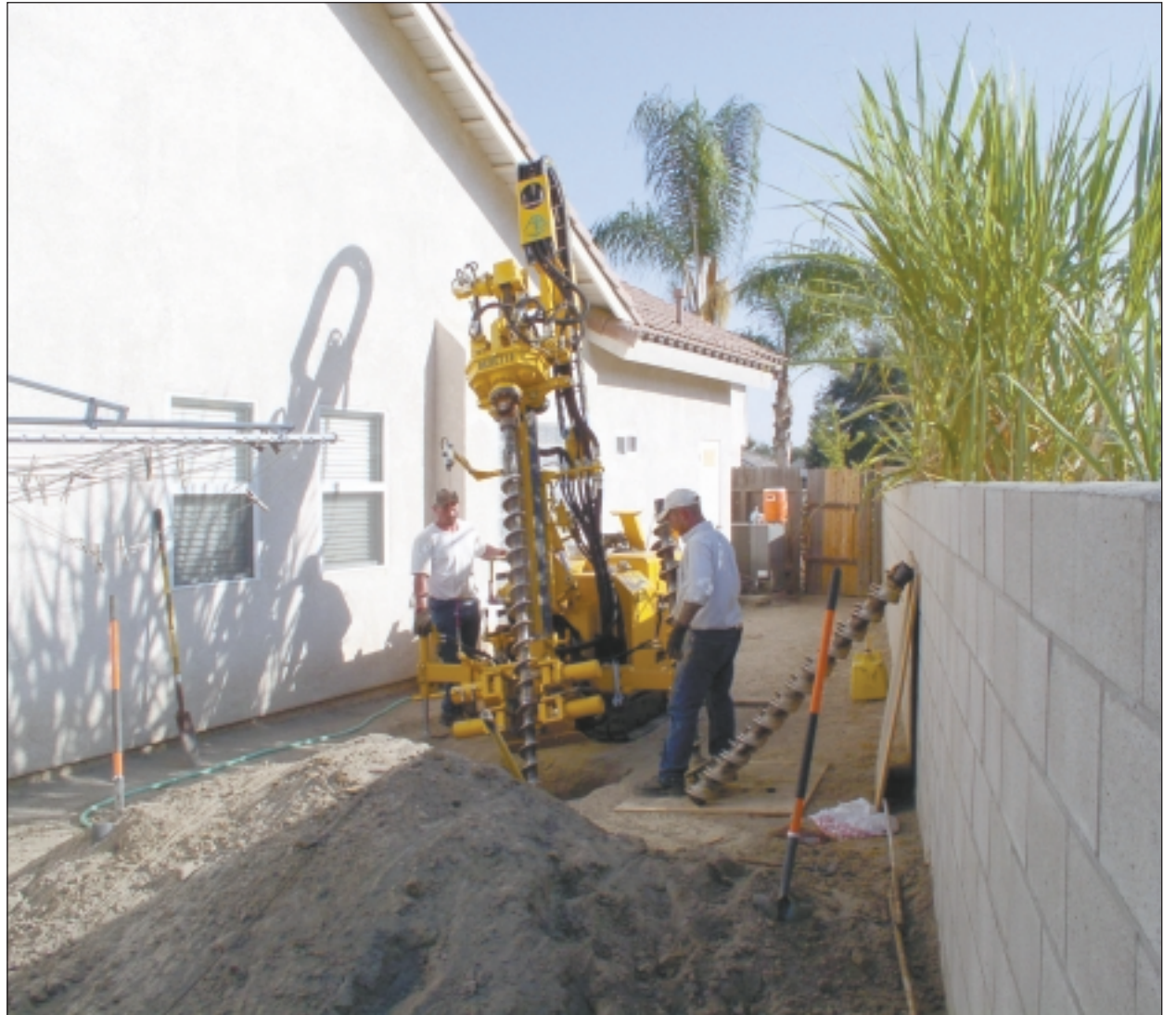
Where ground space is limited, diagonal configurations are common.
