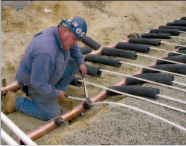
An installer with E.M. Duggan Co., the mechanical contractor tapped to do the installations, crimps a PEX-to-manifold connection.
