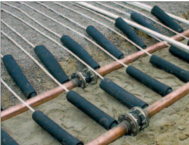
The copper manifold sections were 12 to 20 ft in length. Shown here are flanged expansion joints between sections and sleeves used to keep sand away from valves and fittings, and to permit easier expansion and contraction of tubing.
