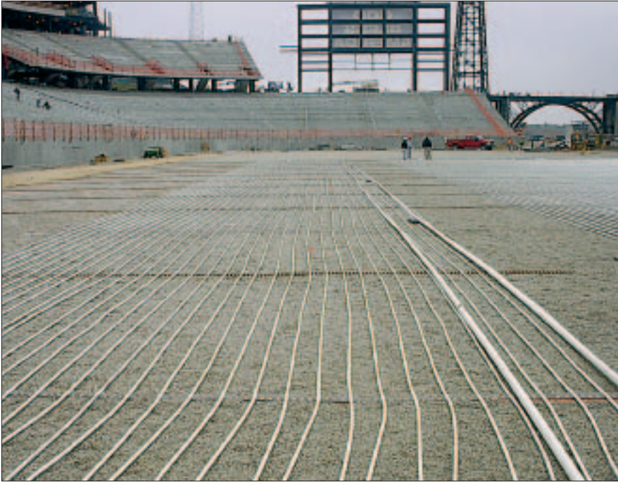
The layout of the tubing is integrated with the larger (right side) irrigation pipe throughout the field's many turf-conditioning zones.
