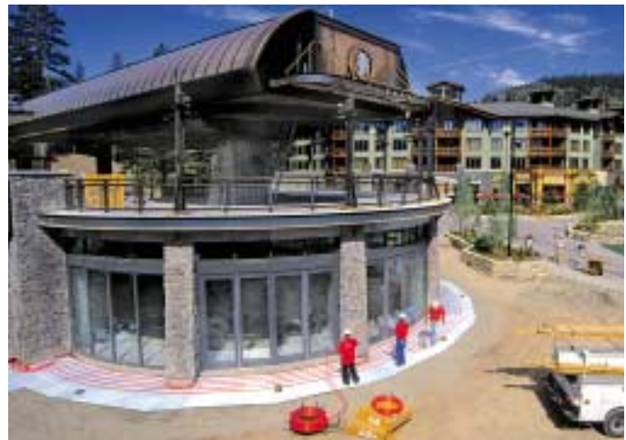
Radiant PEX tubing for snow and ice melting is attached to rigid insulation before layers of sand, gravel and brick pavers at Mammoth Mountain ski resort in Calif.
