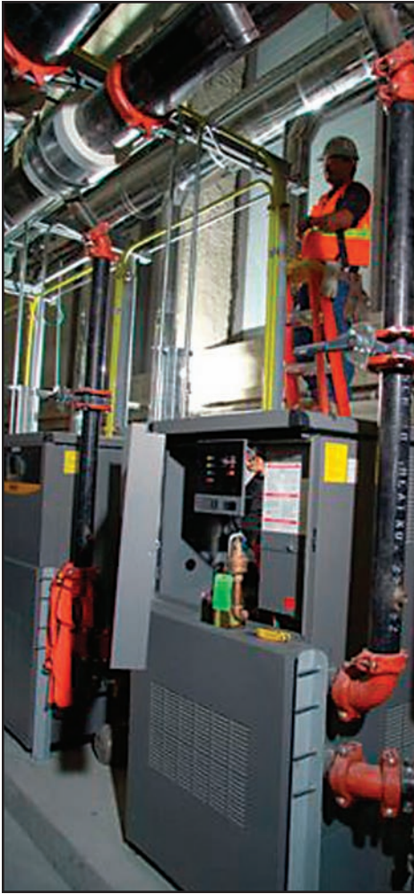
The 10 million Btuh boilers installed in the Phoenix Convention Center feed 58,000 lineal feet of piping to heat the building.
