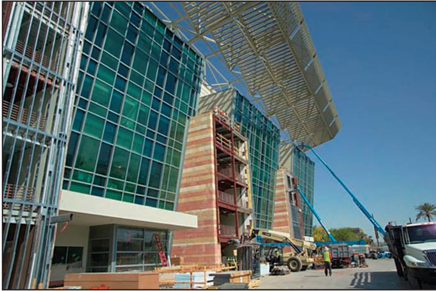
Peel and stick solar panels were used on the exterior of the Phoenix Convention Center to help supply 150,000 kWh annually.
