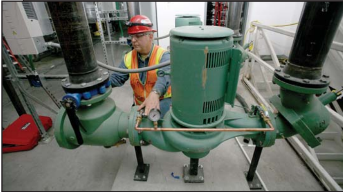
FIGURE 3. An example of an inline pump and drive installation.
