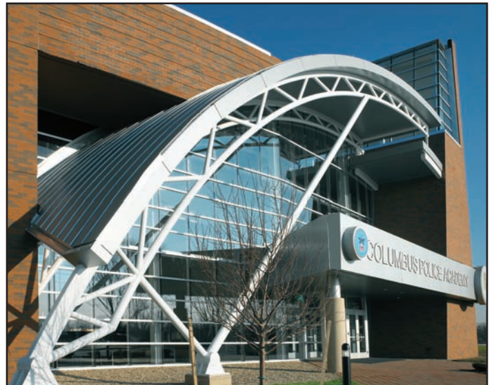
Five-degree angle welds in the pipe were needed to complete the heating loop and accommodate the circular shape of the new police training facility in Columbus, OH.
