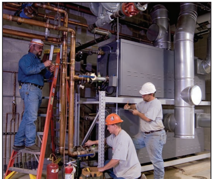
In the mechanical room, four 2-million Btuh boilers, controlled by a BAS and stacked one pair on top of another, provide 16 stages of firing.
