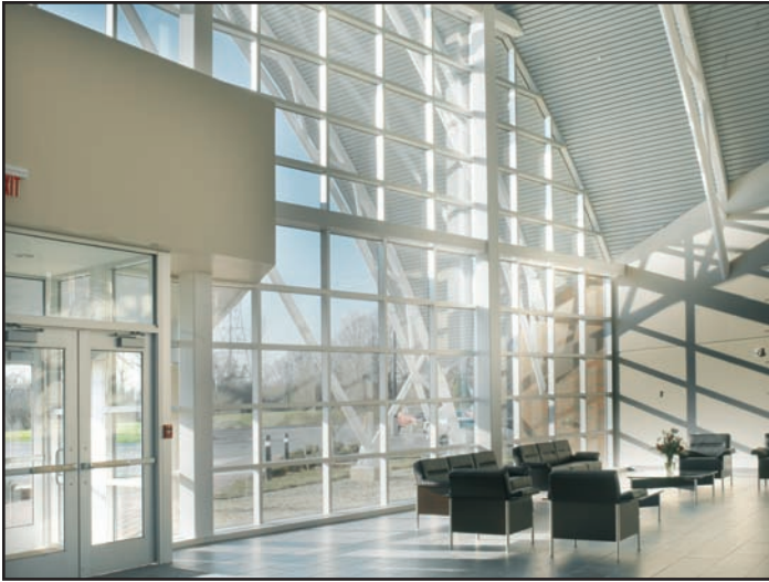
The training facility is heated hydronically with 11 water-to-air heat exchangers that range in capacity from 3,500 to 18,500 cfm.
