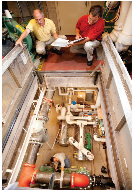
In the bowels of Midtown Exchange are many ClimateMaster water-source heat pumps and several Taco pump stations.
