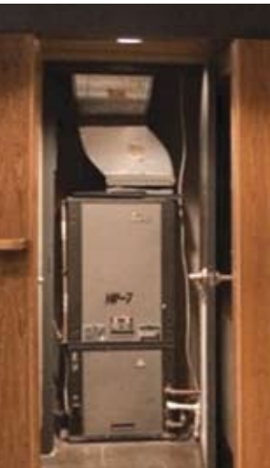
Vertical stacking made good use of limited space in the Alta units.
