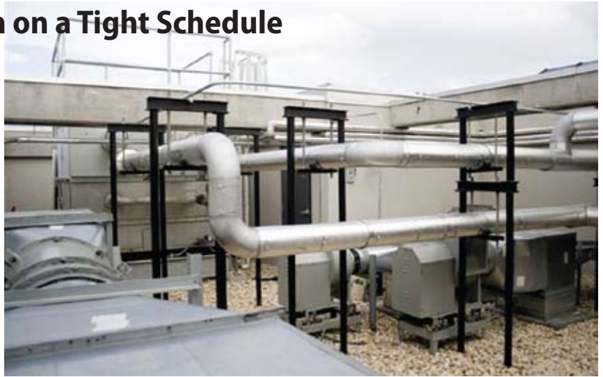
In addition to the extensive mechanical system, the Alta development's roof was incorporated with green roof elements to reduce urban heat, and to enhance on-site storm water management.
