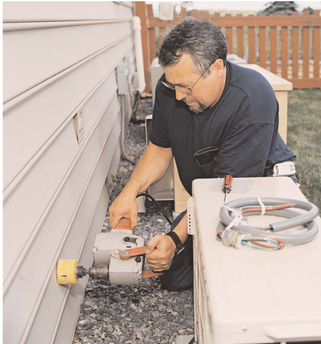
Dave Yates drills a hole in the garage wall through which he will run a refrigerant lines to the outdoor unit. Since the system uses R-410a refrigerant, it can run at a higher pressure and the line sets can be smaller.
