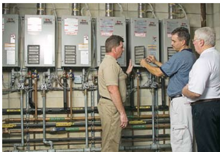
Service manager Paul Webb of Sun Plumbing explains the operation of the new manifold of recently-installed tankless water heaters.
