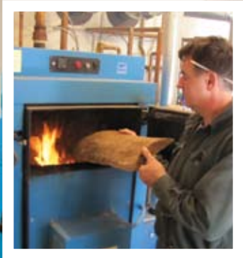
Merv Wenger loads hardwood into the Econoburn boiler.
