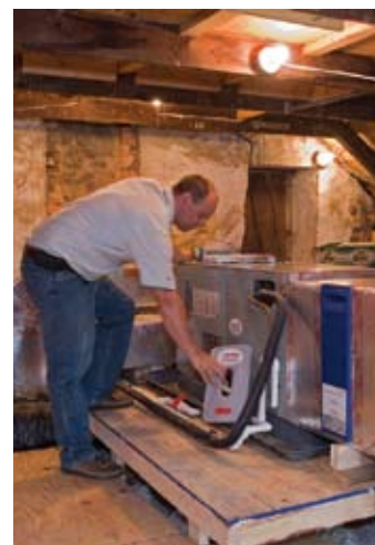
Vince Youndt checks the air handler section of the system.
