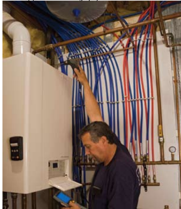
Dave Yates uses a Testo to perform a combustion analysis of the wall-hung boiler as the job nears completion.
