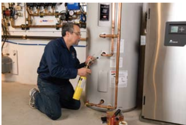
Dave Yates makes a sweat connection between the “geothermal boiler” and the indirect water heater.
