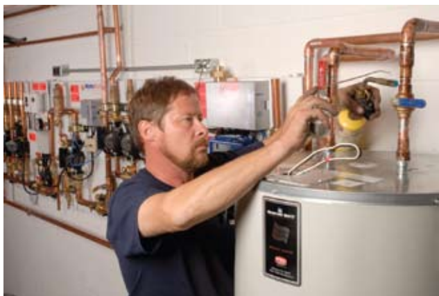
Bob Sieger connects one of the two twin-coil Bradford White indirect water heaters.
