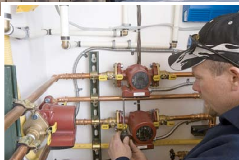
The radiant system features a control panel and several Grundfos multi-speed circulators.
