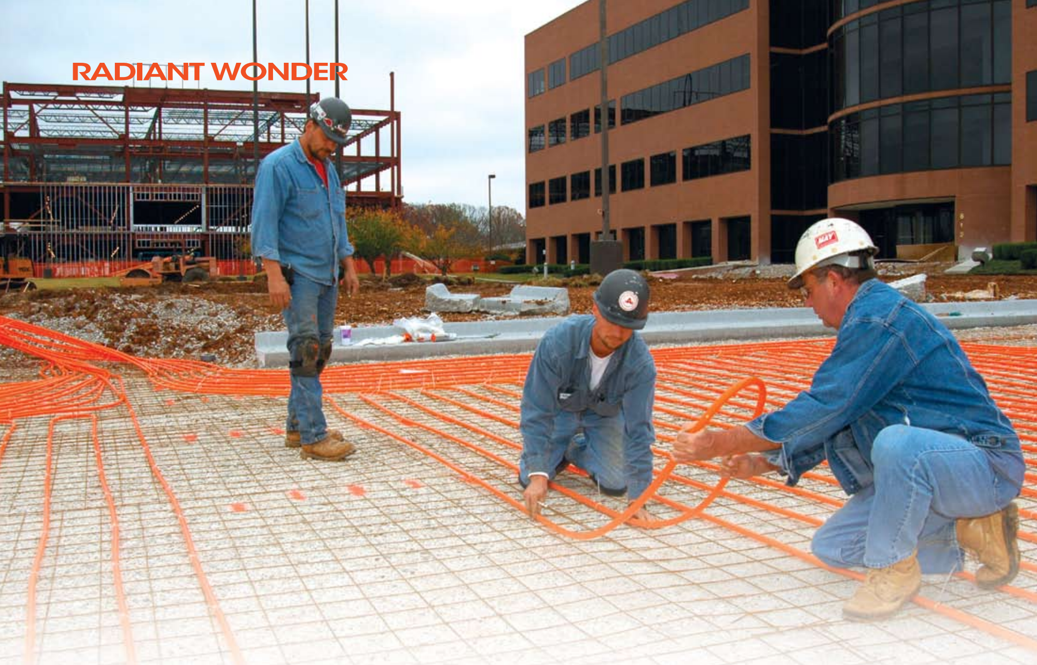
Employees from Action Inc. install one of the many loops for the extensive snowmelt system at the new J.B. Hunt facility.
