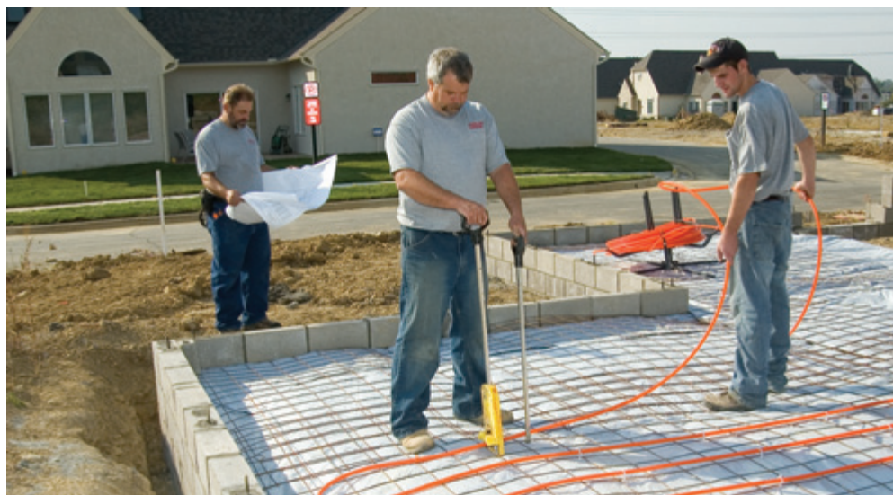
Flex tubing goes into the floors to heat from below.
