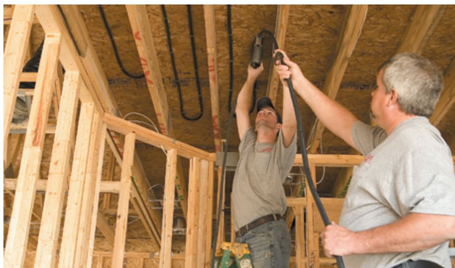
Pipes in the ceilings provide radiant comfort.
