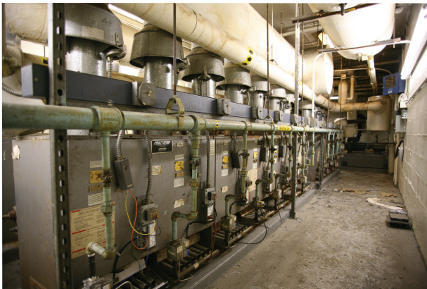
Before the retrofit, Spring Creek Gardens' main boiler room had 22 400-MBh cast-iron atmospheric boilers, several of which fed heat to indirect-gravity domestic-hot-water tanks.
