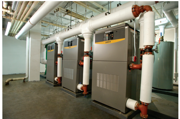
One of Spring Creek Gardens' six new boiler rooms. This one includes three fully modulating, 2.2-million-Btu Rheos+ boilers to meet space- and domestic-water-heating needs.
