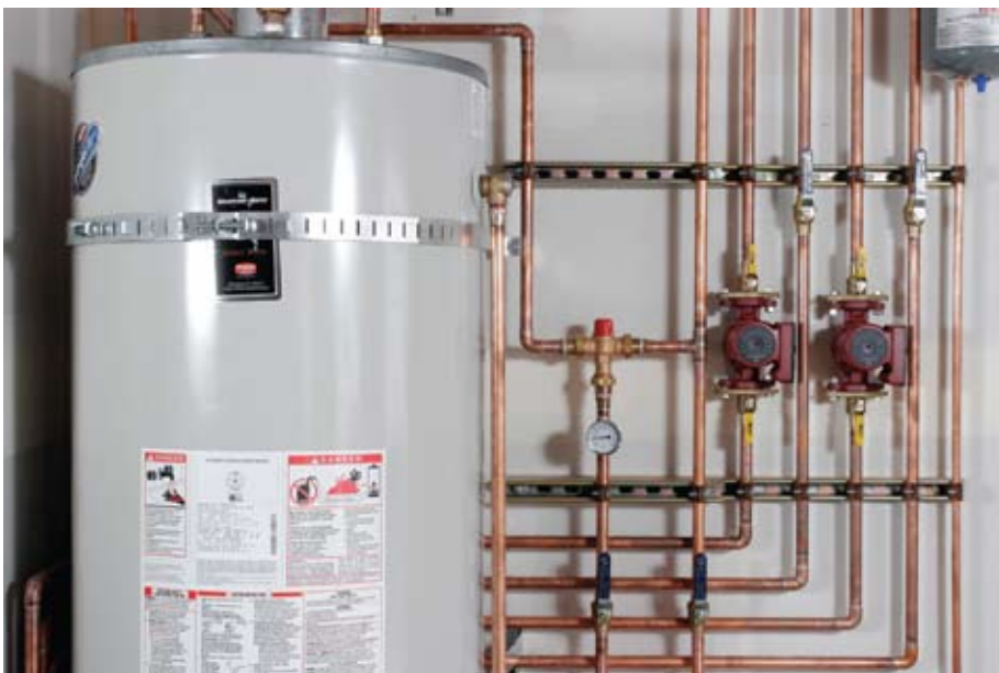
Components from Bradford White, Watts and Grundfos are part of radiant hydronic heating systems, Statewide style.
