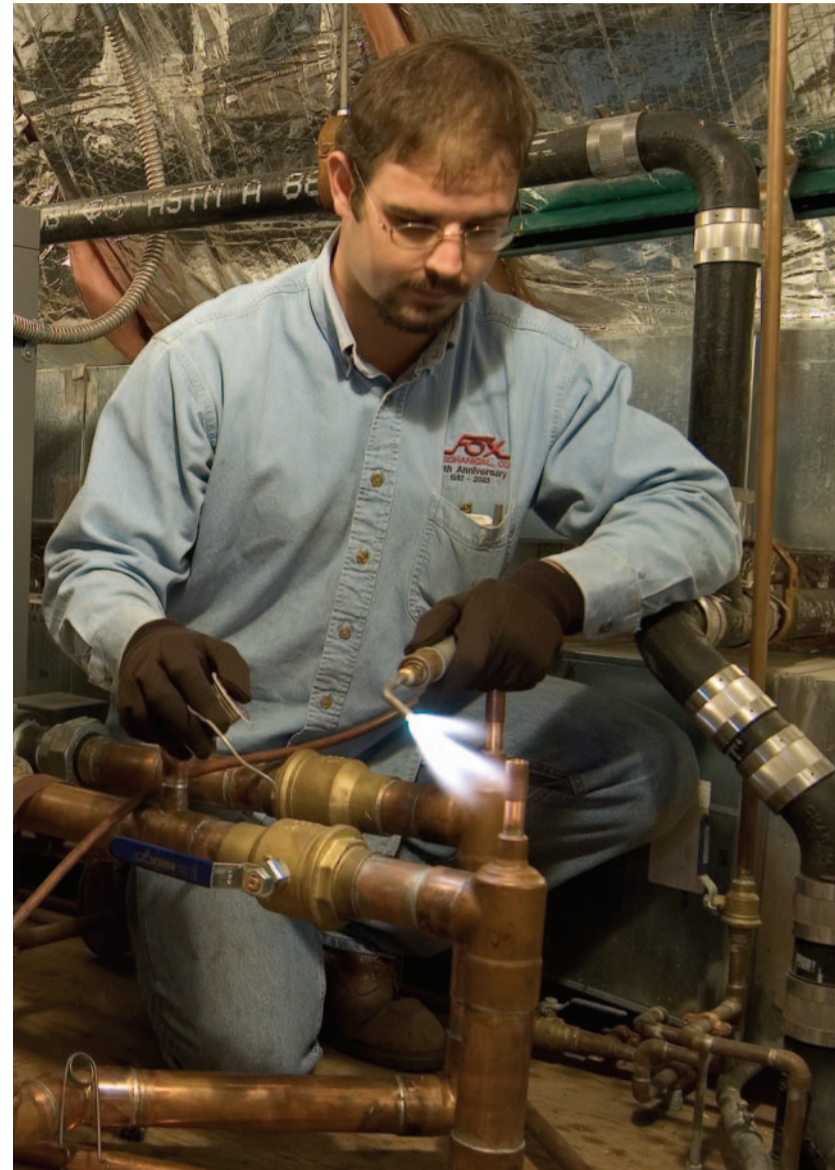
Tim Kaiser sweats a connection during final installation of the 500 MBH, sealed-combustion Laars Pennant system.
