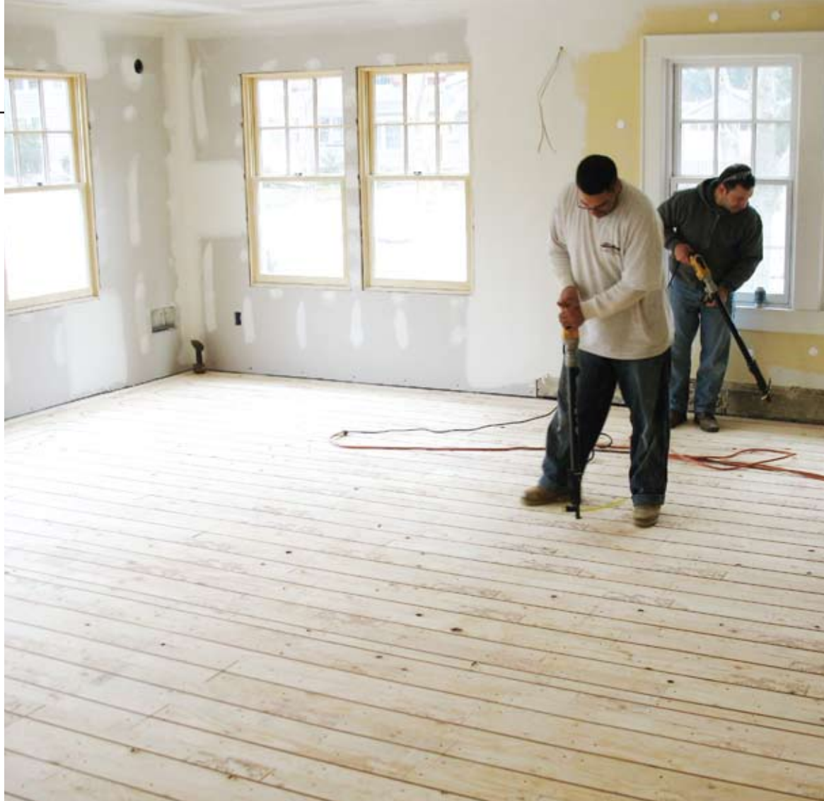
In this home, Greg Jannone retrofitted an existing steam system, converting radiators from steam to hot water and installing radiant heating over the first floor and new master bathroom.
