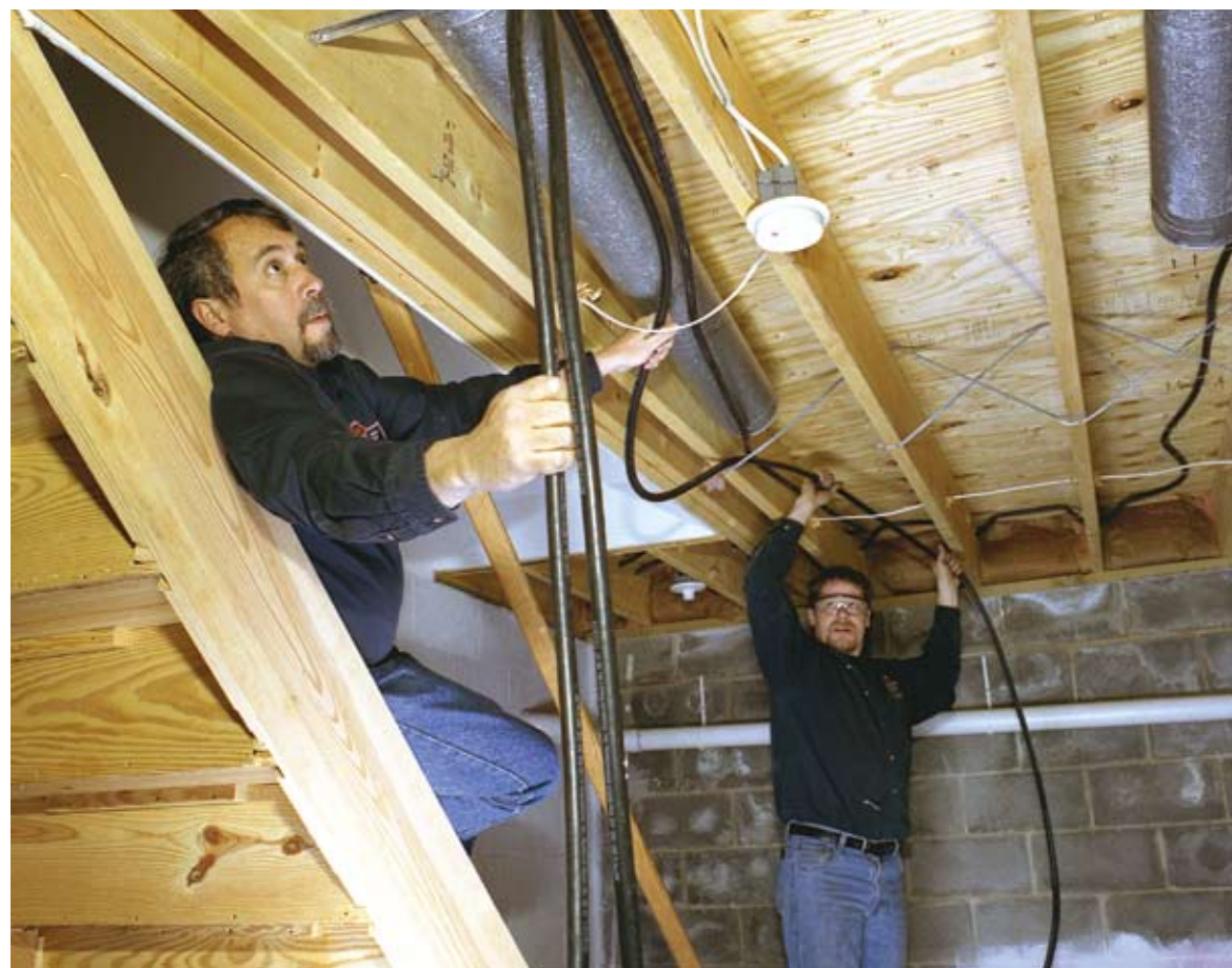
Dave Yates (foreground) and senior technician Bob Sieger slide Onix tubing into place for joist bay staple-up. The tubing is flexible and can be pinched to go through holes.
