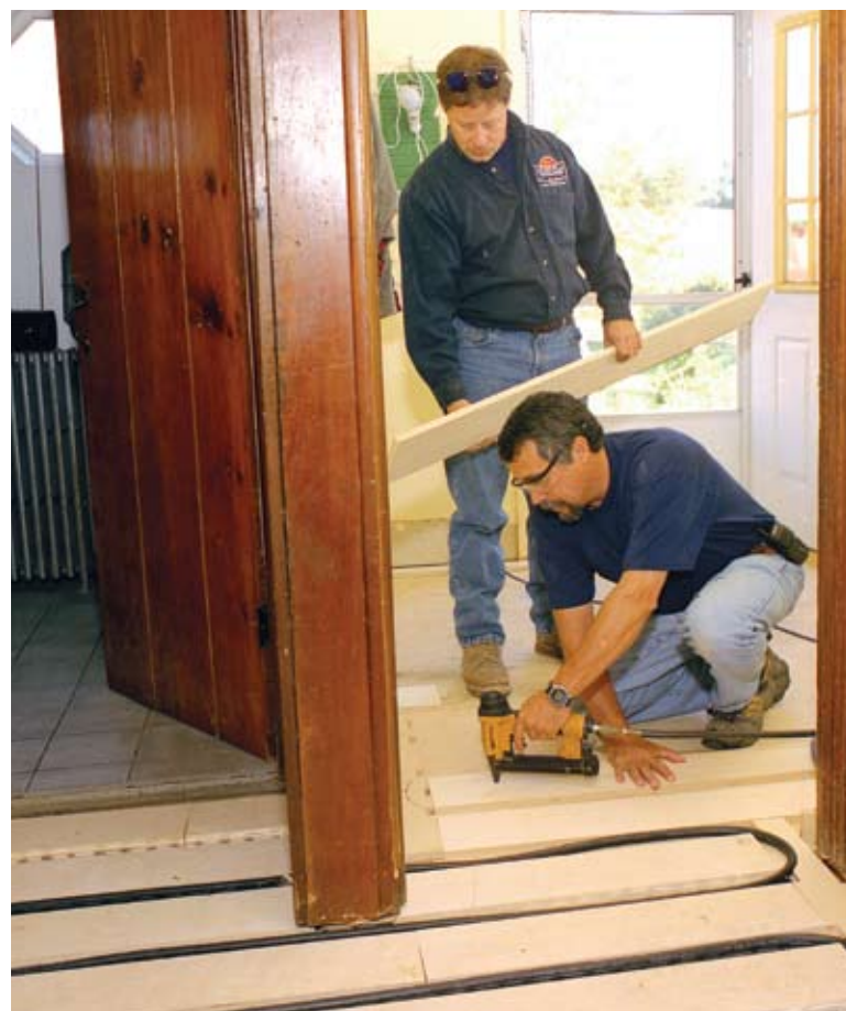
Dave Yates (foreground) and senior technician Bob Sieger complete a SubRay installation as part of an extensive radiant retrofit.
