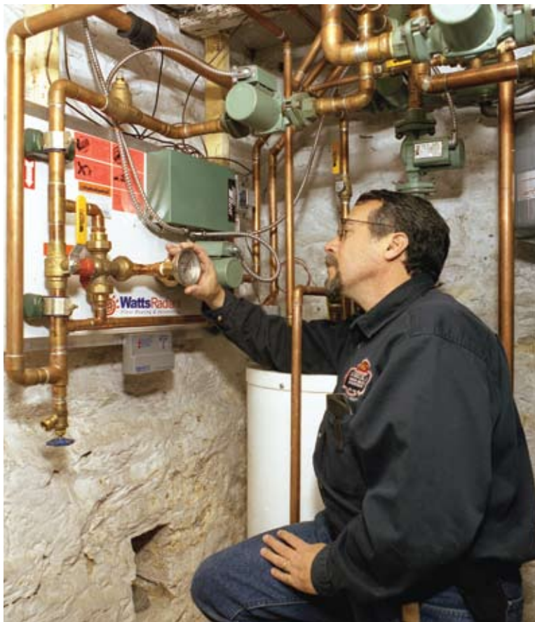
Dave Yates checks system performance during pre-fire at a residential radiant heat retrofit. He used Hydronex panels to reduce time on the job site.
