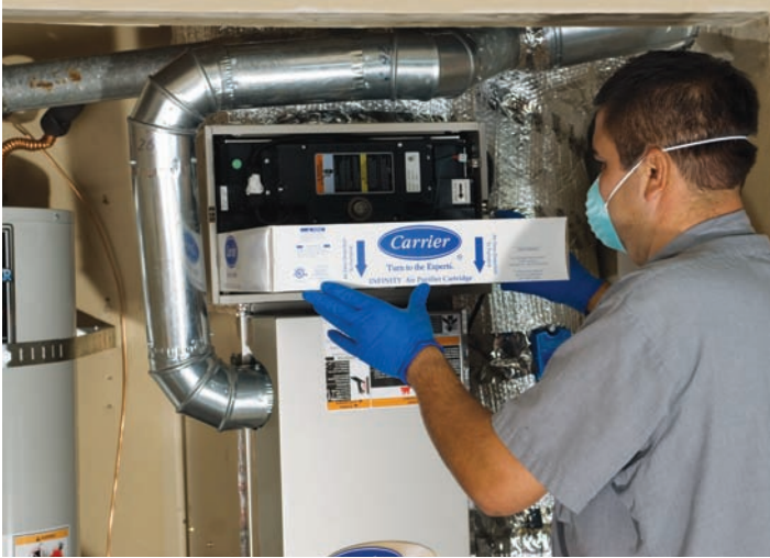
Sal Gonzalez, service technician at ABC Cooling, installs a replacement filter bag for an Infinity Air Purifier.
