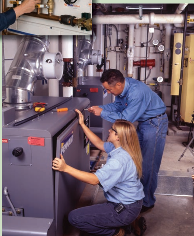
Shoreline Community College, Seattle, replaced all boilers with high-efficiency units by Laars.
