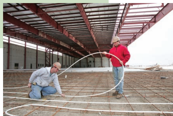
Watts Radiant PEX tubing is installed as part of a hydronic heat system.
