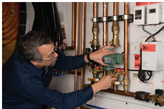
A contractor puts a Taco circulator on a Watts Radiant Hydronex panel.
