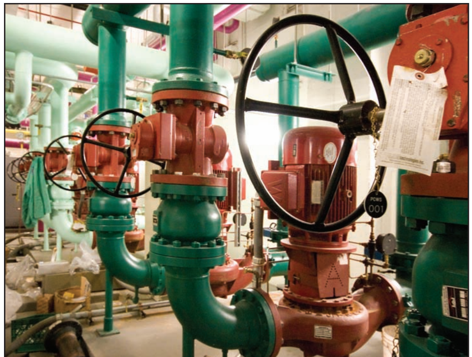
The multiple condensing boiler/cooling-tower arrangement for the closed-water-loop heat exchange system is physically, part of the tower's energy-efficient design.
