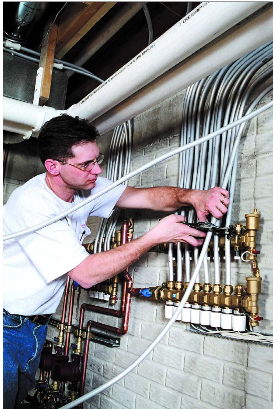
Mark Krumnow, a radiant heat and hydronics controls expert with manufacturer's rep firm, MBA Corp., designed the radiant heat system and installed the FAR control package, which manages radiant and forced air systems in one simple, five-zone controller. Radiant heat is controlled as the primary source of heat with forced air as the secondary source of heat.
