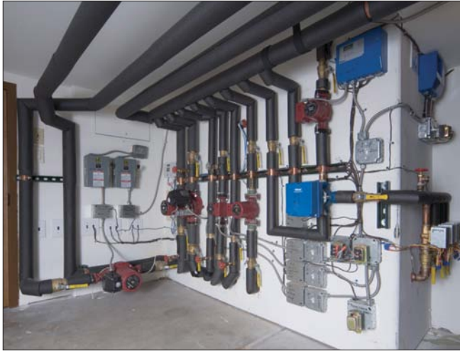
Concept Mechanical designed this system with several multispeed circulators for maximum flexibility and control. (Photo courtesy of Grundfos Pumps.)
